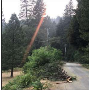
Figure 4: Image of Vegetation Related Damage in Nevada County – Falling Treetop Damaged Primary Overhead Conductor and Broke Crossarm
