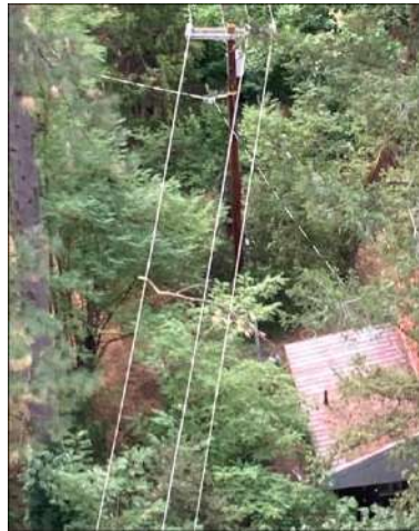
Figure 5: Image of Veg Related Hazard in Sierra County – Tree Branch Caught in Multiple Overhead Phases
